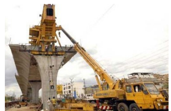
More such projects need to undertaken by the Government in collaboration with the Private sector to make projects more viable
